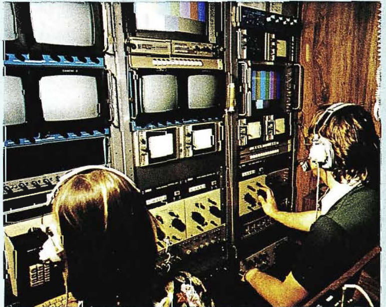
Graphics and video-control operating positions in front of monitor, test and distribution racks.
