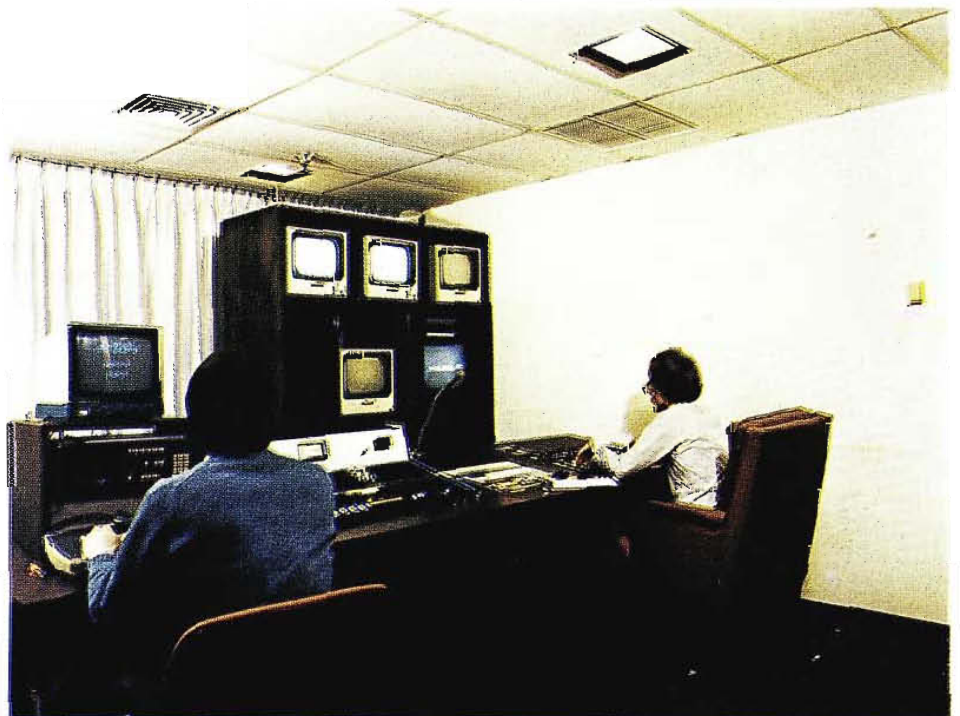
Production control center adjoins studio, with complete facilities for audio and video switching; character generator; camera controls; distribution.
